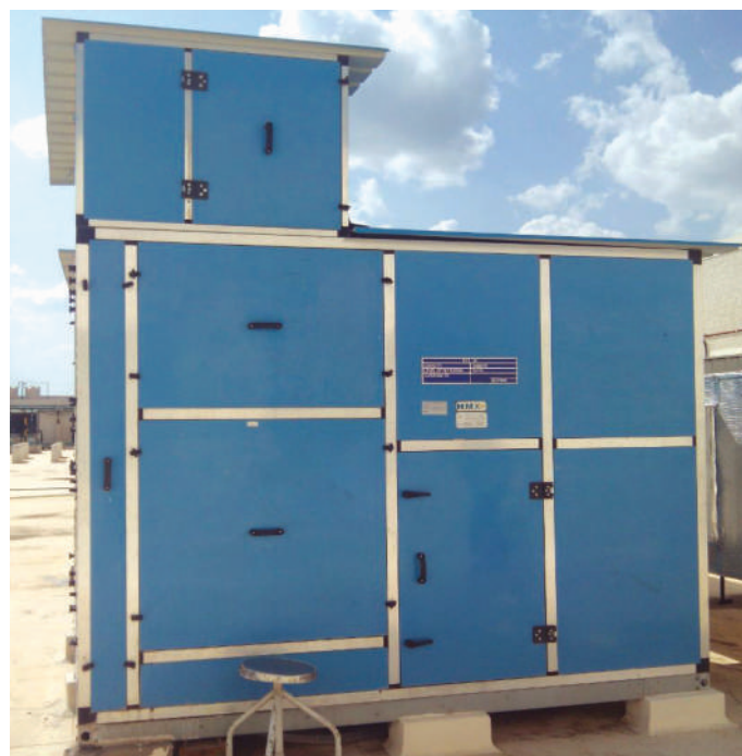
HMx-IDEC of 15,000 CFM capacity installed at Himalaya's Bangalore plant
