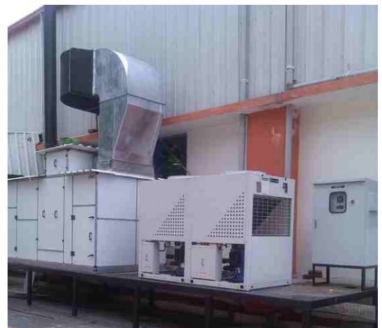
HMX-PCU-F at the site
