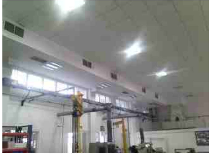
Ducting layout inside the carbide grinding floor
