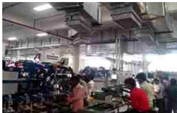
Ducting layout inside the factory
